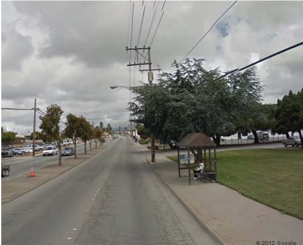
Bus Shelter and failing pavement on east side of Freedom Boulevard in front of the Santa Cruz County Health Services Agency offices
