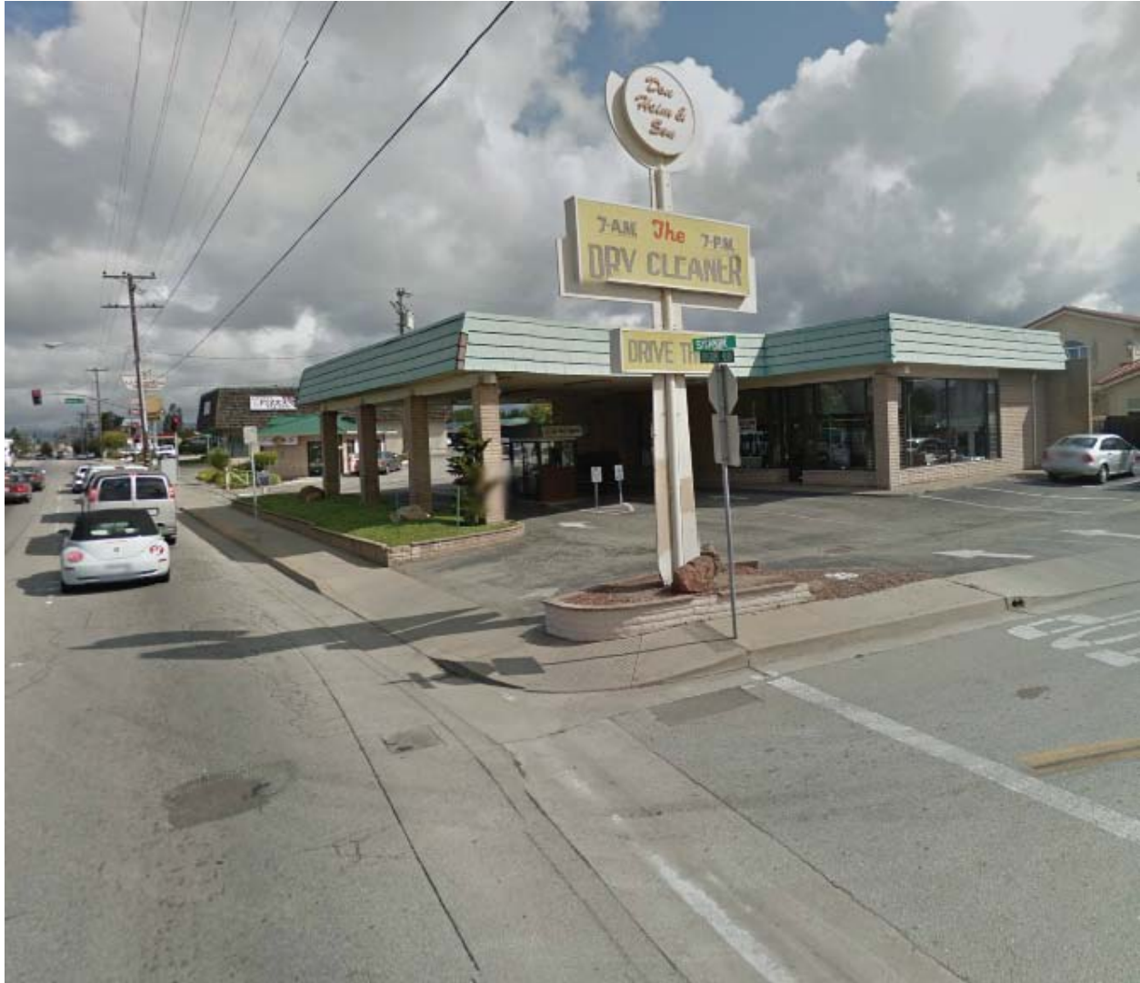
Non-compliant ADA compliant ramp and driveway and failing asphalt at northeast corner of Freedom Boulevard and Sycamore Street
