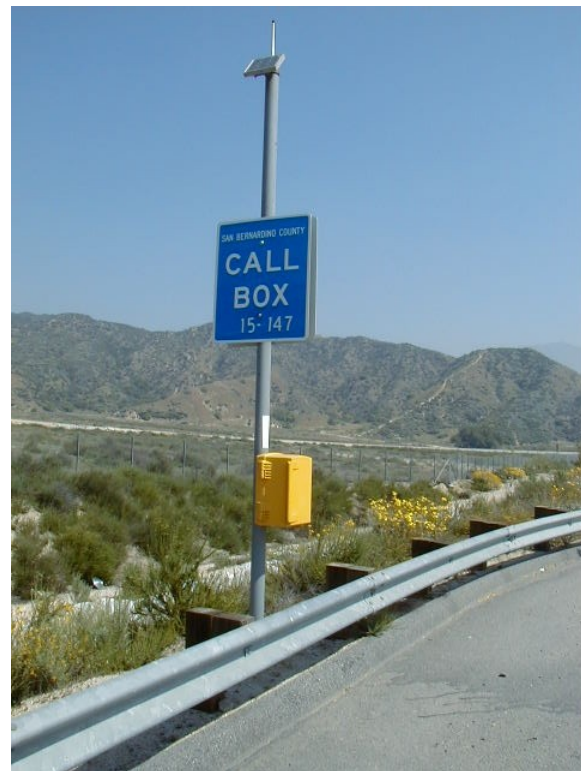
Site Type F – installed behind a guard rail.
