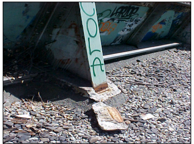
Spalling at Base of Guardrail
