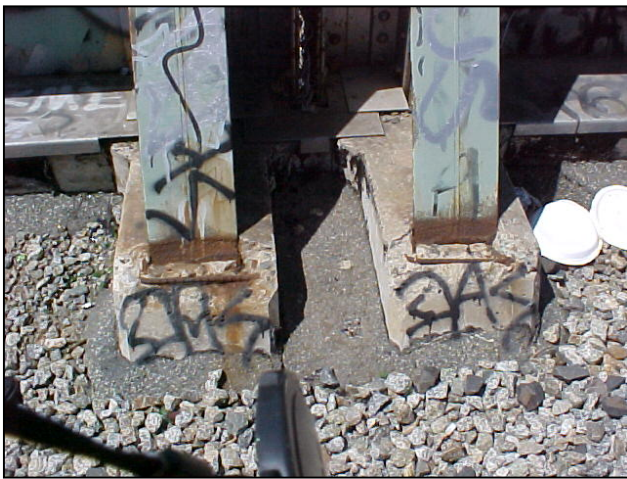
Spalling of Concrete Base at Guardrail Stiffener Support
