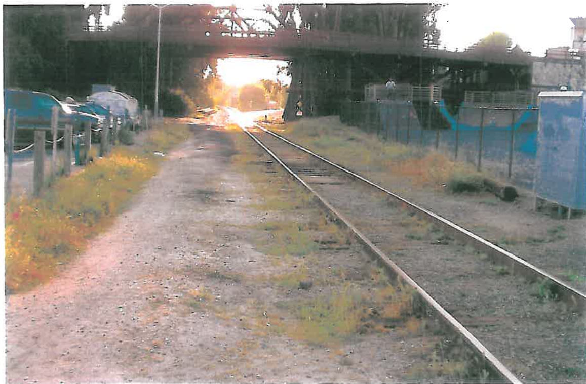
RR looking west from Pacific Street and under W. Cliff Dr bridge. Wye to right behind bridge.
