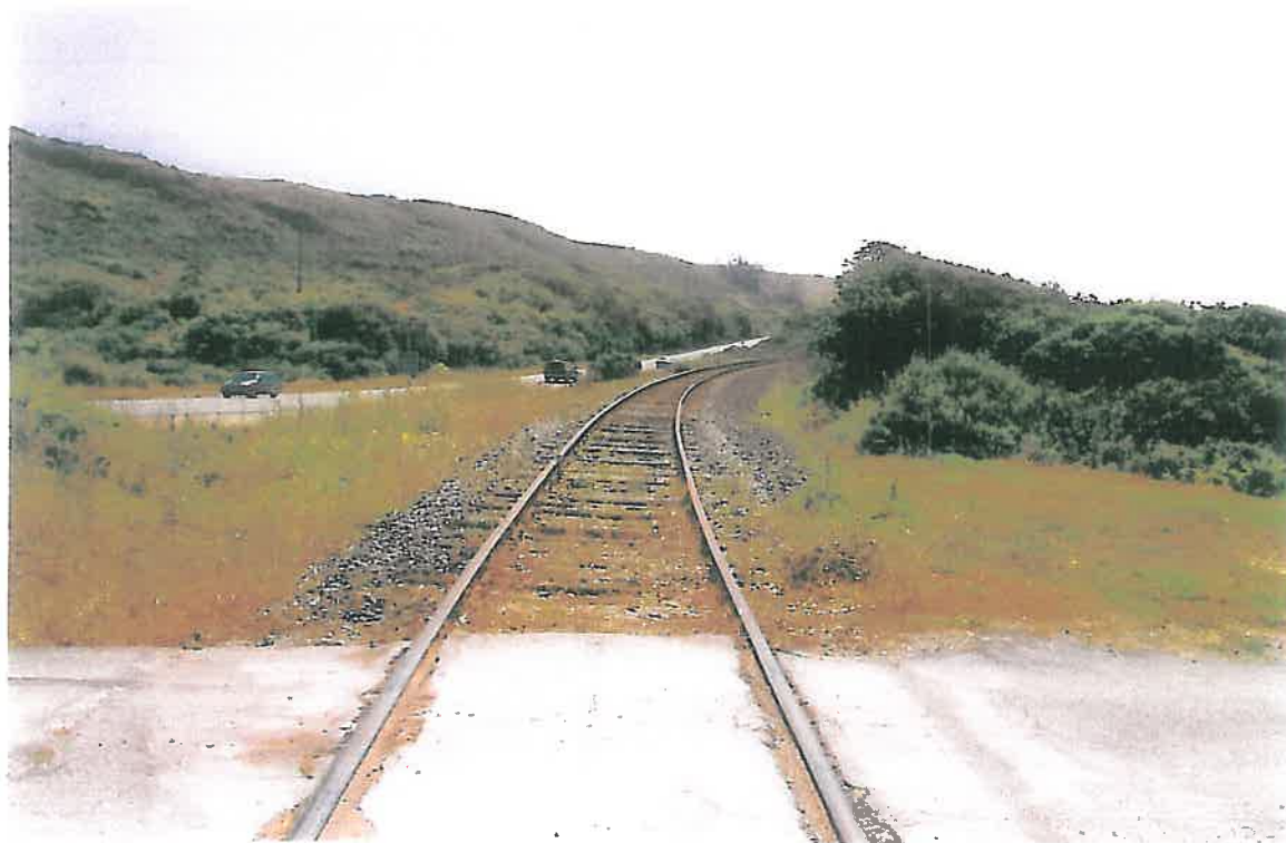
RR looking SE across north crossing of Scaroni Rd (Hwy 1 adjacent in background)
