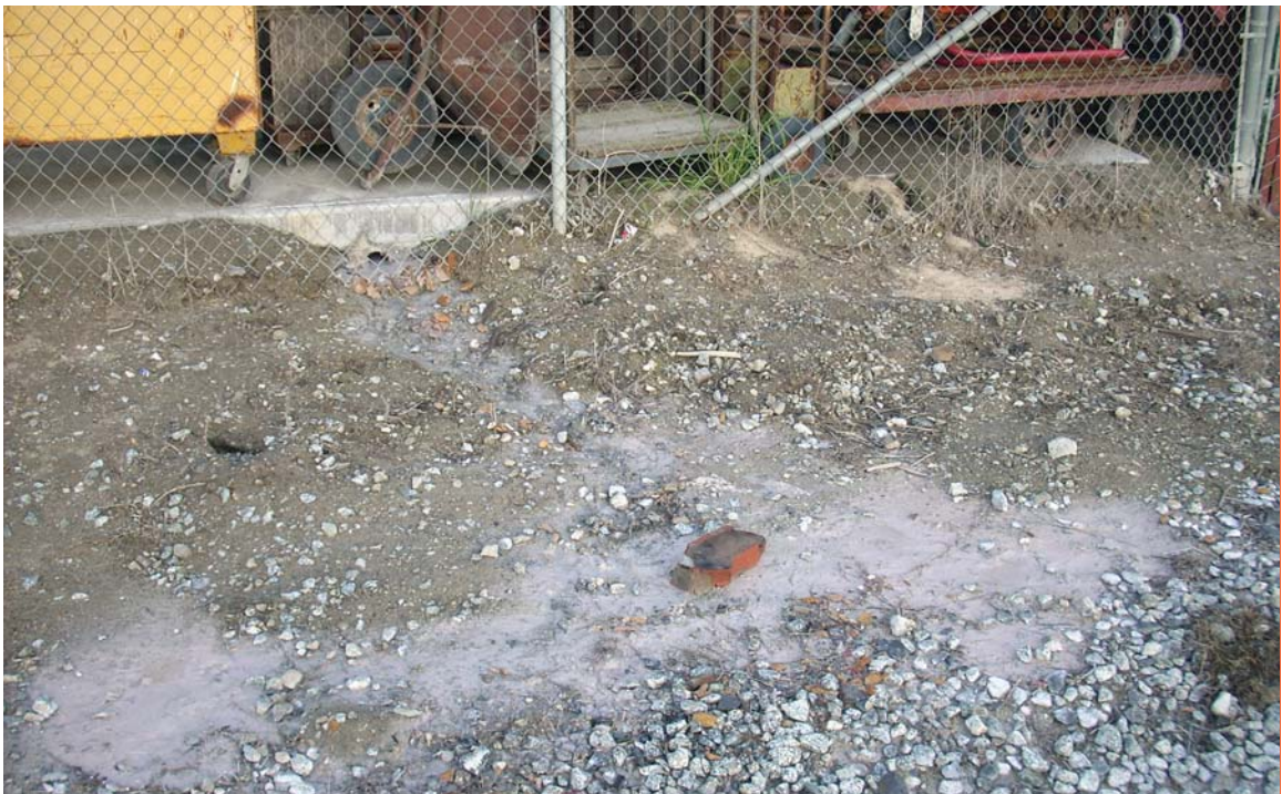
Photograph 2. Runoff from Gino Rinaldi, Inc. property near SB-96. View to east from the Branch Line.
