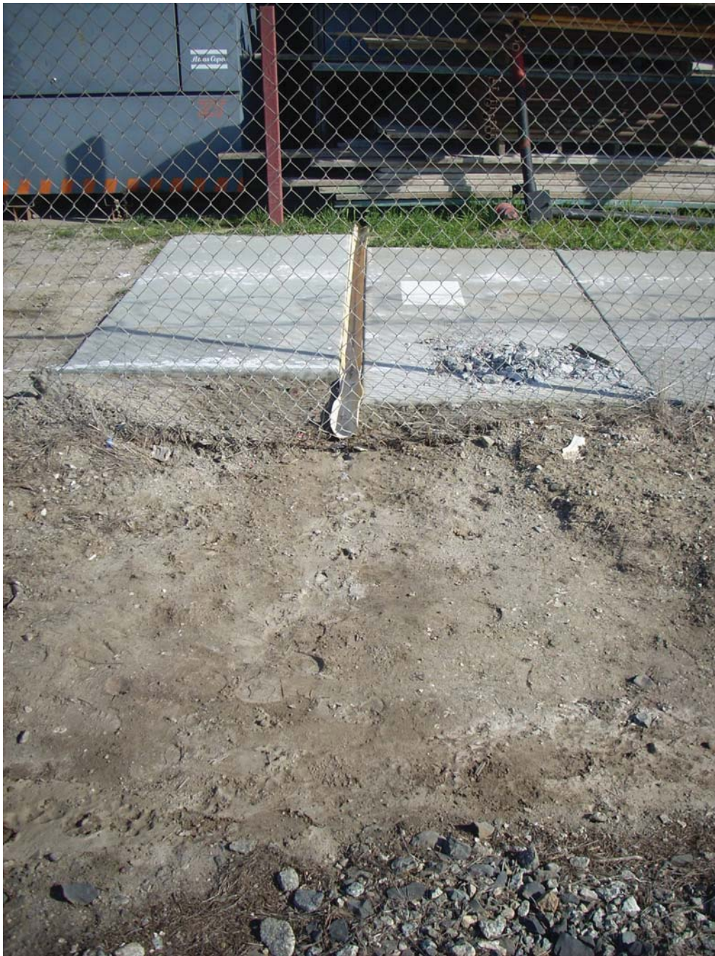
Photograph 3. PVC drainage pipe at Gino Rinaldi, Inc. property near SB-95. View to east from the Branch Line.
