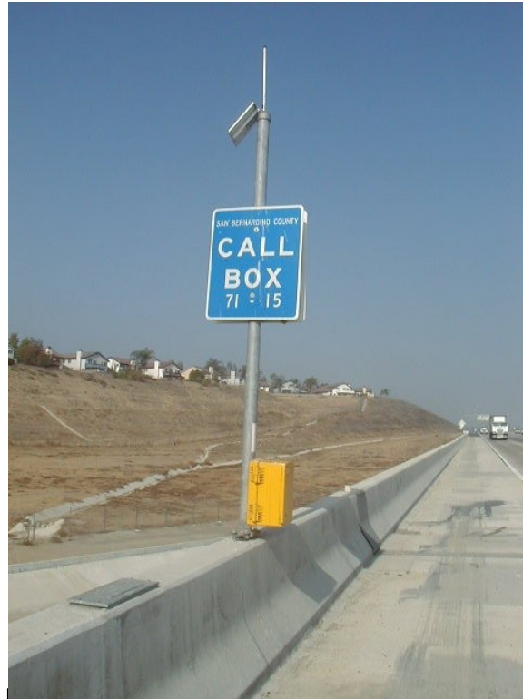
Site Type H or K – installed on a k-rail or concrete barrier.
