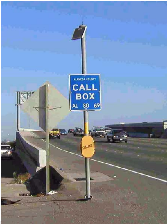
Site Type G – installed at-grade, in concrete.
