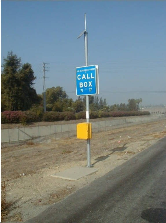
Site Type A – installed at-grade, in soil.
