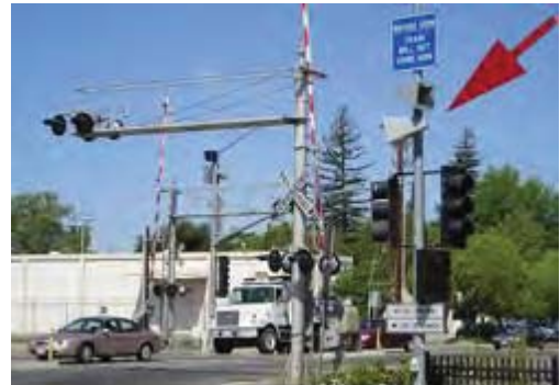
Wayside Horn. Source: City of Fort Collins
