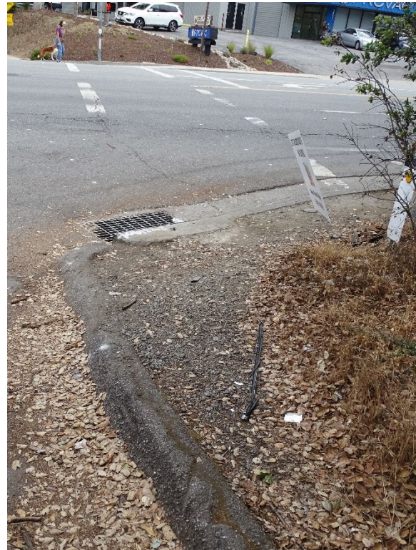
Lack of ADA compliant curb ramp
