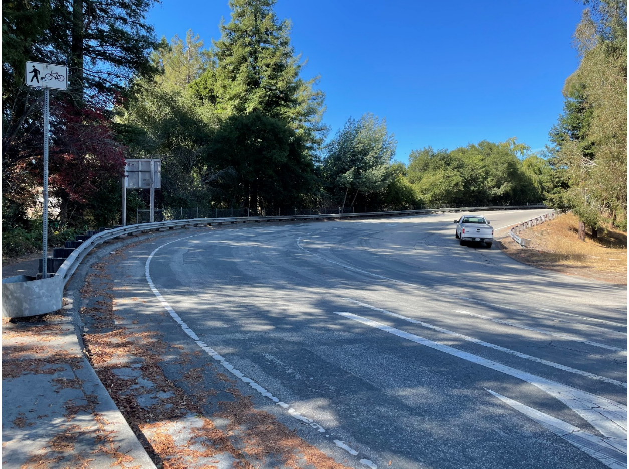
Figure 4 Right turn lane bicycle conflict point to be addressed with bicycle striping improvements
