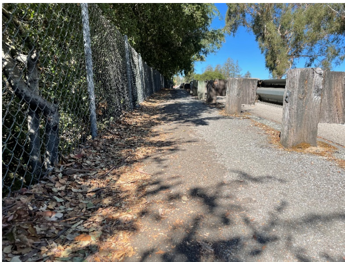
Figure 1 Pathway Patching and slippage
