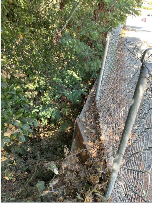
Figure 2 Retaining Wall Failure
