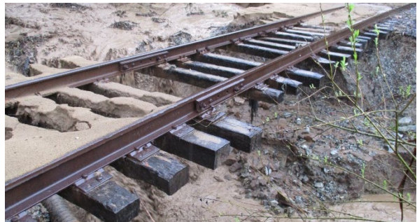
Damage to the Santa Cruz Branch Rail Line because of flooding during 2017 storms
