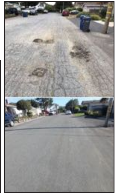
Before and after road resurfacing, County of Santa Cruz. Above: Santa Cruz Avenue. Left: Riverside Drive.
